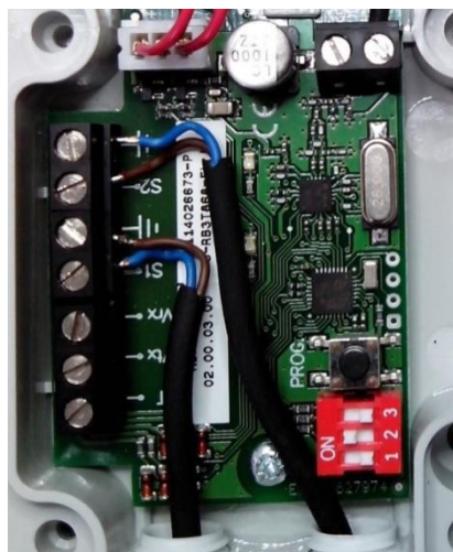
Illustration 17: Example connection of safety contact strips to the JCM RB3R86 transmitter
